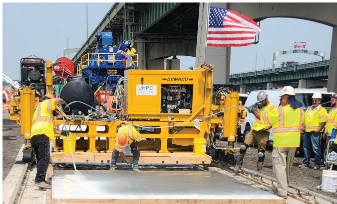
The GOMACO UHPC paver demonstrated its capabilities at the 2023 International Symposium on Ultra-High Performance Concrete in Wilmington, Delaware.
